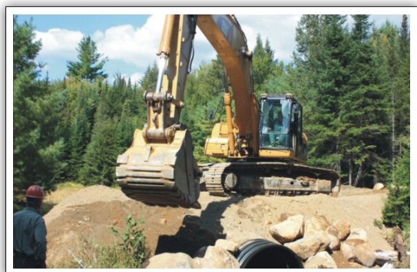
5. Build up backfill on both sides, compacting the native material with the excavator bucket. Cross over as soon as minimum fill cover is achieved.
